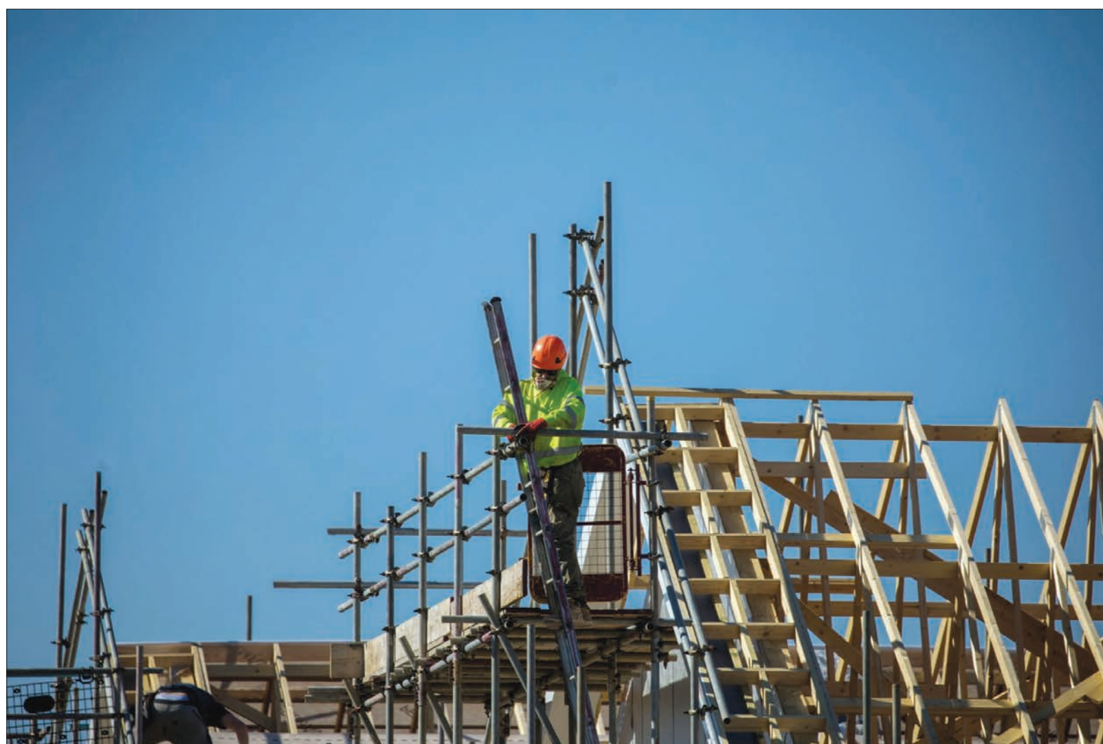
A workman stands on scaffolding support on a residential property building site in Harwich, UK. Data yesterday showed UK construction activity suffered its sharpest slowdown since 2009 last month — despite the sector being spared a national lockdown.
